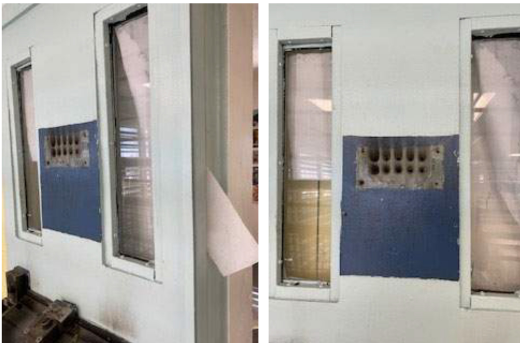
Figures 1, 2 – Mr. Ubiera’s Cell Window (Right Side) as Photographed by BOC Staff on August 23, 2023
